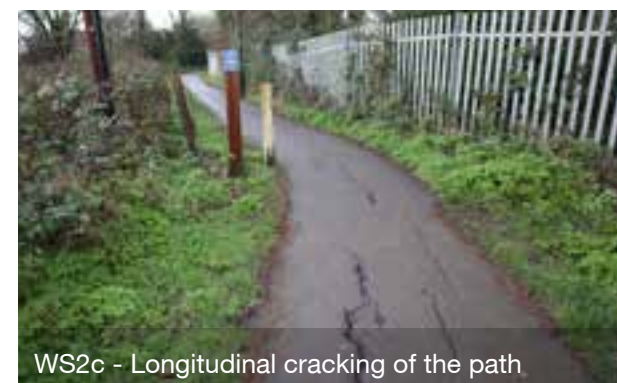
WS2c - Longitudinal cracking of the path.
